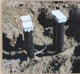
Cascade School Four Salcor 3G UV Units connected in a parallel/ series array
