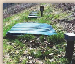
Mud River Project Over 50 Salcor 3G UV Units installed with ANUA peat filters.
